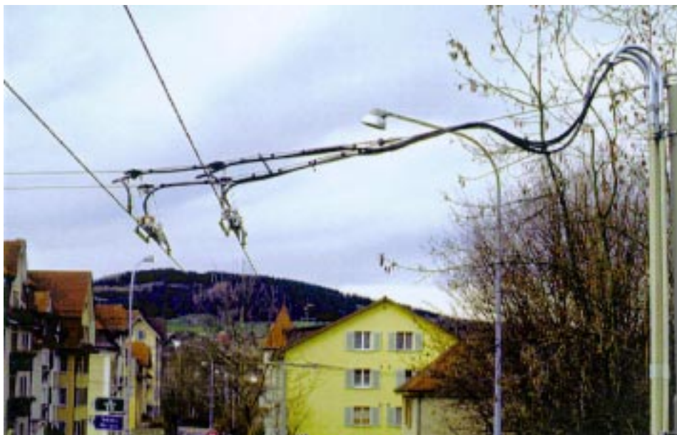
Figure 3.3.4 Feeder point with section insulator (Source: Furrer+Frey).
